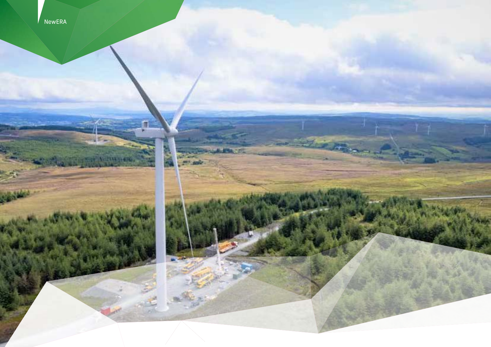
▲ Final turbine installation at Lenalea Wind Farm, Co. Donegal, co-development by Coillte and SSE Renewables.
